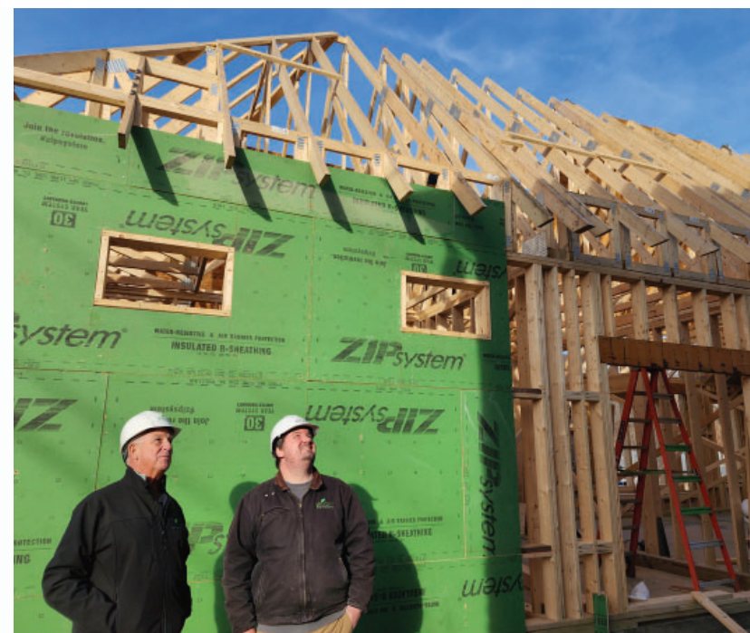
CELEBRATING 50 YEARS AS WESTERN NEW ENGLAND'S LEADER IN SUSTAINABLE AND HIGH-PERFORMANCE RESIDENTIAL, COMMERCIAL & INSTITUTIONAL CONSTRUCTION
